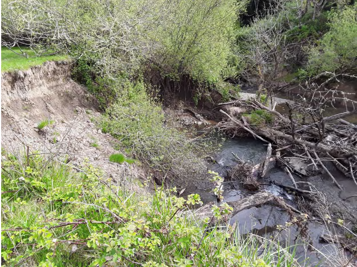
Figure 24: Example area within reach 1 that has a natural structure creating fish habitat, however it also appears to be assisting in the bank erosion near a pasture. Other design options would include reshaping the bank 1:1, setting the fence back, and replanting.
